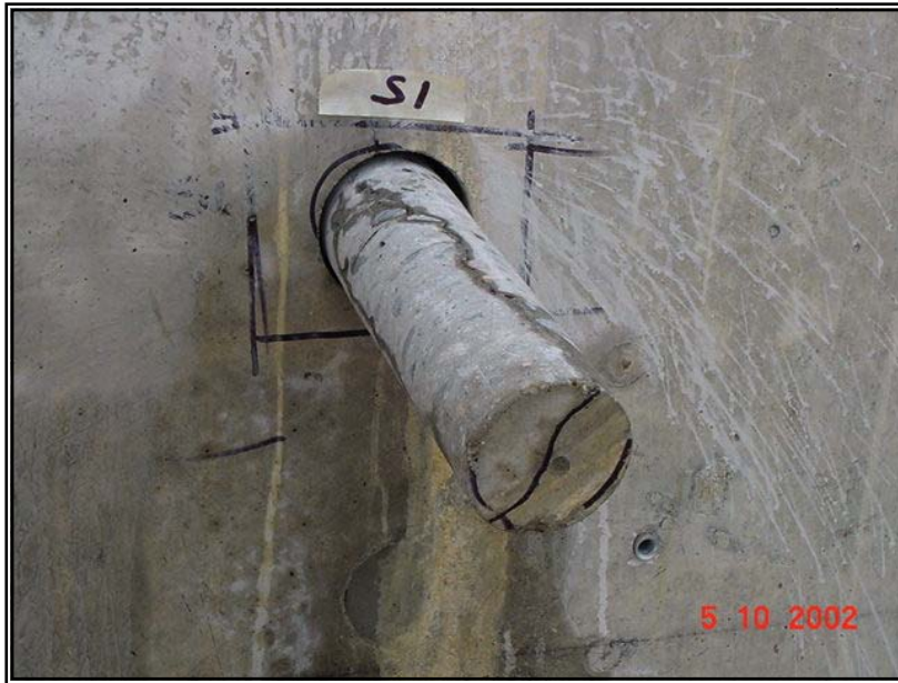
A 75mm diameter core containing a crack at wall 1 was extracted for laboratory analysis.
