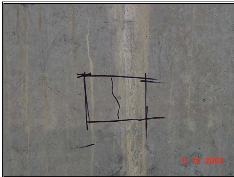
The location of sample S1 extracted at the cracked area on wall 1.
