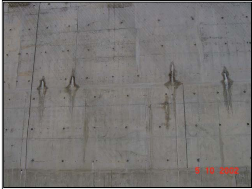
Sign of efflorescence with water marks were noted on wall 3.
