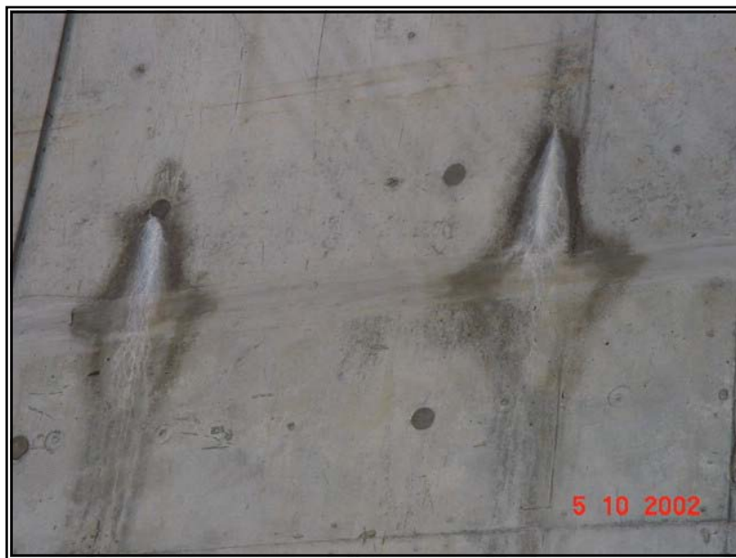
Close view of the sign of efflorescence accompanied with water marks were noted on wall 3.
