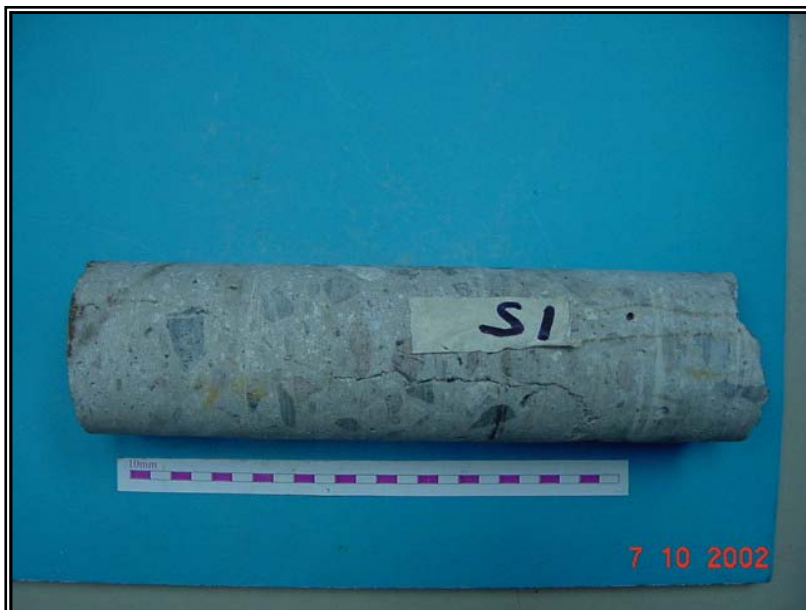
A crack perpendicular to the exposed surface was seen in core S1.
